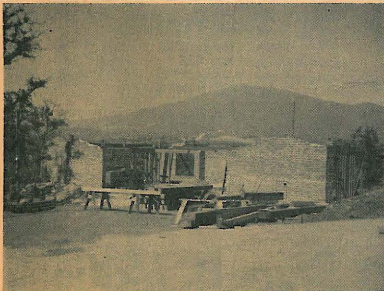
Construction is well underway on the new home being built by Ben and Ruth Polak on Palo Verde Ranch. The new home is being constructed of adobe brick in traditional style with modern touches of large windows. The site is on the hill south of the entrance to Palo Verde and commands an imposing view to the north and east looking down on the lake. Echo Photo.
